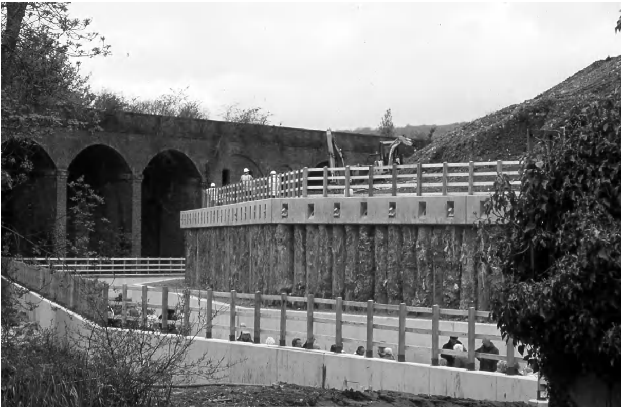
Fig 2. Capel's Mill Stroud canal diversion: Another view of the public taking the never to be repeated opportunity to walk in the new channel. The height of the old tip retained by the concrete piles may be clearly seen in the top right hand corner.
