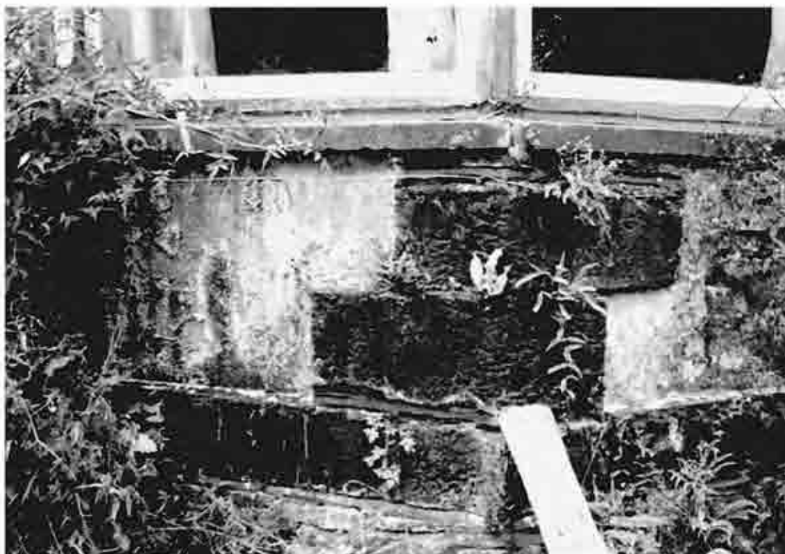
Figure 12. Angle-ended, bay type rectangular copper slag blocks at Highbury Farm, Redbrook, Newland
