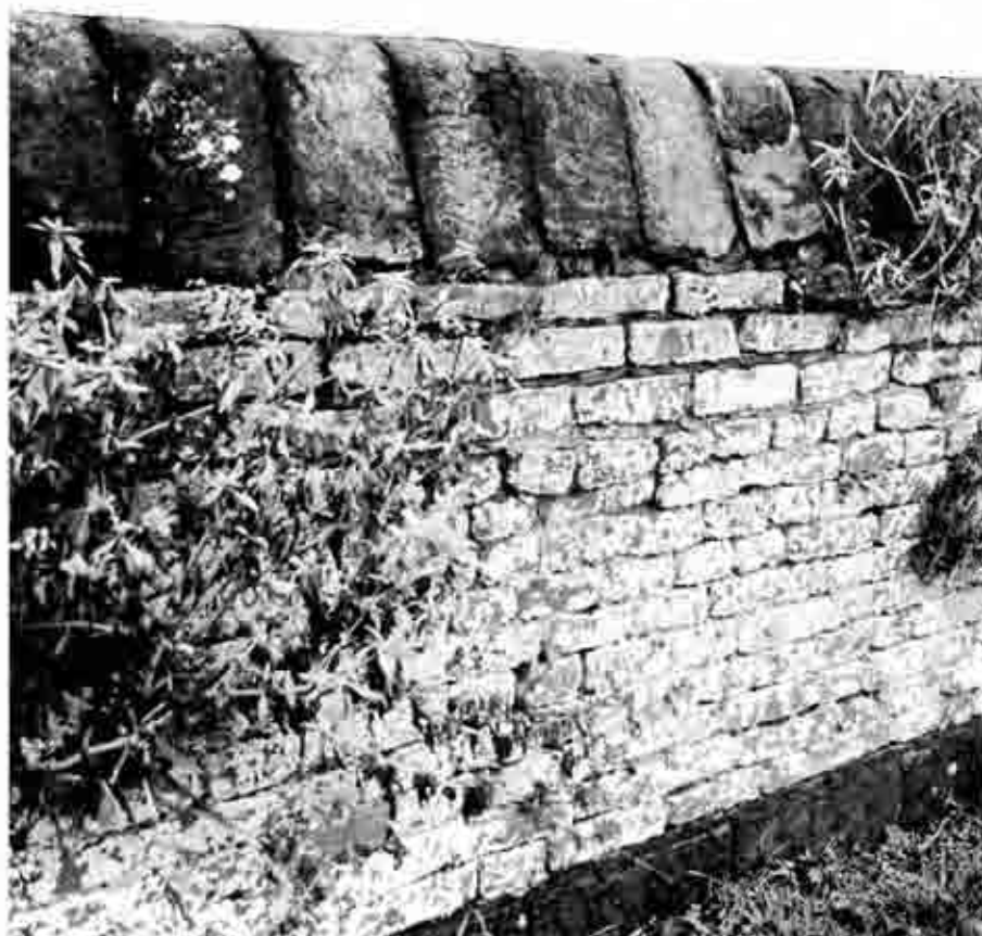
Figure 9. Triangular copper slag blocks used as wall copings at Nastend House, Nastend, Eastington,
